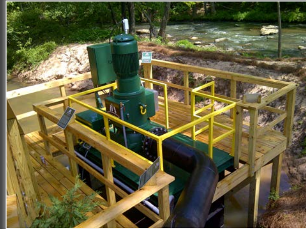
VFH Turbine™ and public observation deck before flooding.
