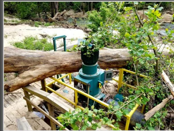
VFH Turbine™ was 18ft. under water.
